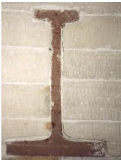
Fig. 1 End view of cast iron beam: note bubbles in cast iron, variations in flange thickness
